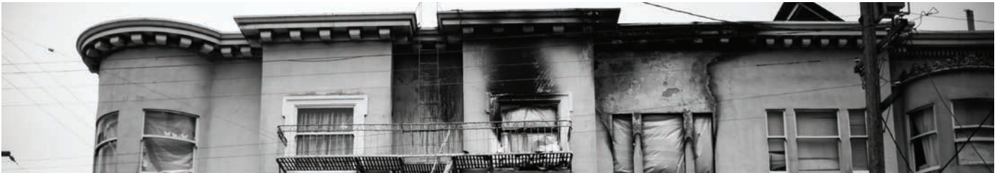
PHOTO: Damage to residential building at the corner of Baker and Hayes Street. Photo Credit: Joseph Wilinski. www.joewilinski.com
